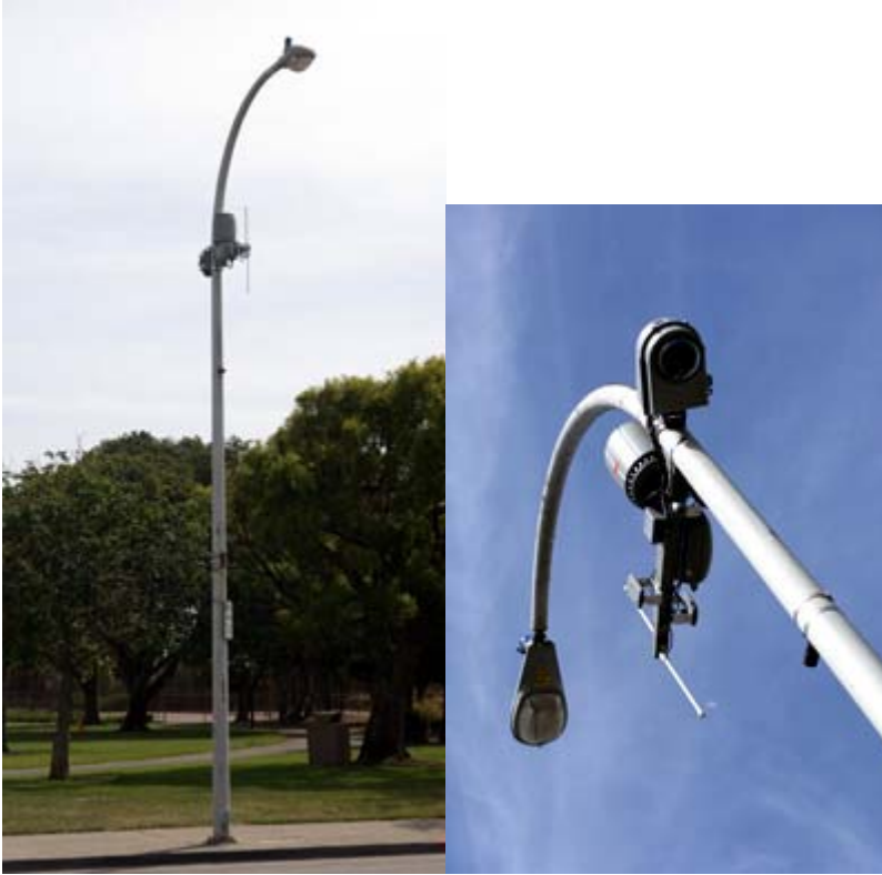
CAPTION: A pan-tilt-zoom camera and BelAir units on a telephone along MacDonald Avenue beside Nicholl Park.
